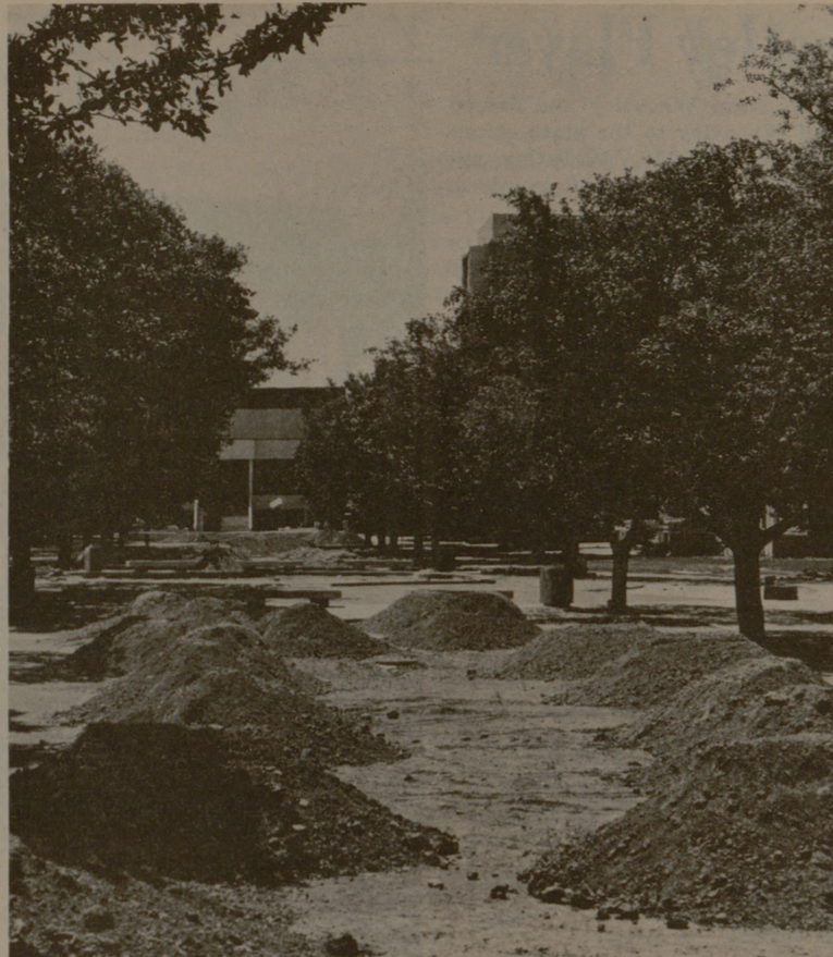
GIANT MOLES HAVE TAKEN OVER A&M— Not really, but with mounds and mounds of dirt scattered about due to the intense campus construction, they may as well. This picture was taken near the new $20 million MSC complex center. (Photo by Peter Leabo)
