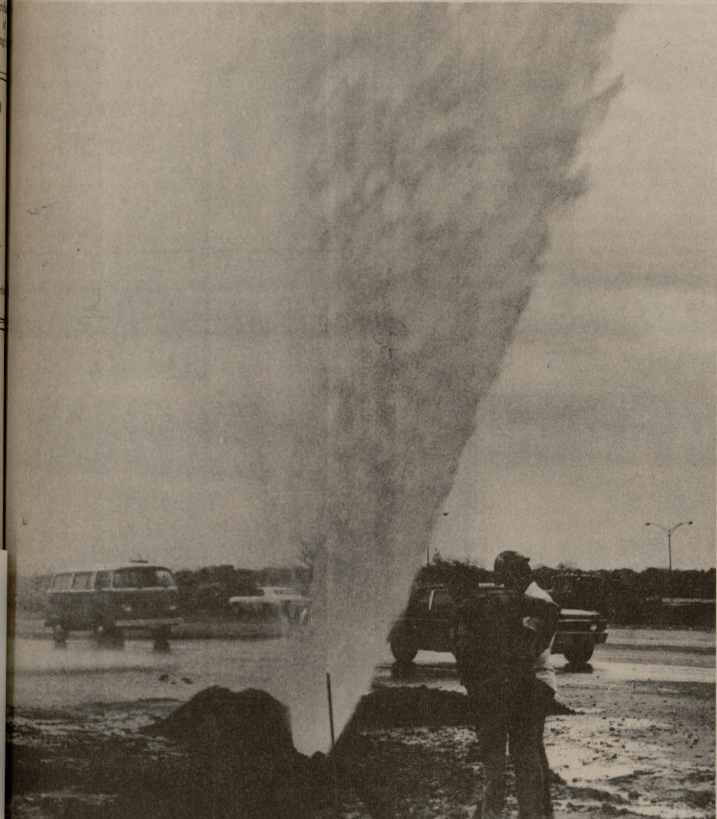
WORKING LIKE A GEYSER in eruption, a 12-inch water pipe let loose with all its Tuesday afternoon at the corner of S. College Ave. and Bizzell St. where workers digging a cable canal for stoplights being erected at the intersection. Job superintendent Don Hartman of the Alder Electric Co. said initial plummage of the 'geyser' about 100 feet and took about 45 minutes to shut off.
