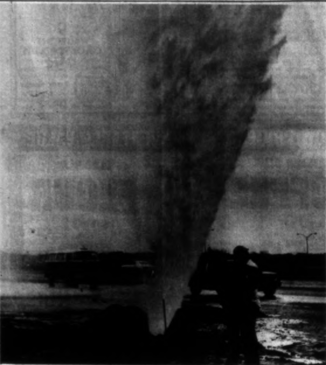
LOOKING LIKE A GEYSER in eruption, a 12-inch water pipe let loose with all its fury Tuesday afternoon at the corner of S. College Ave. and Bizzell St. where workers were digging a cable canal for stoplights being erected at the intersection. Job superintendent Don Hartman of the Alder Electric Co. said initial plummage of the 'geyser' was about 100 feet and took about 45 minutes to shut off.
