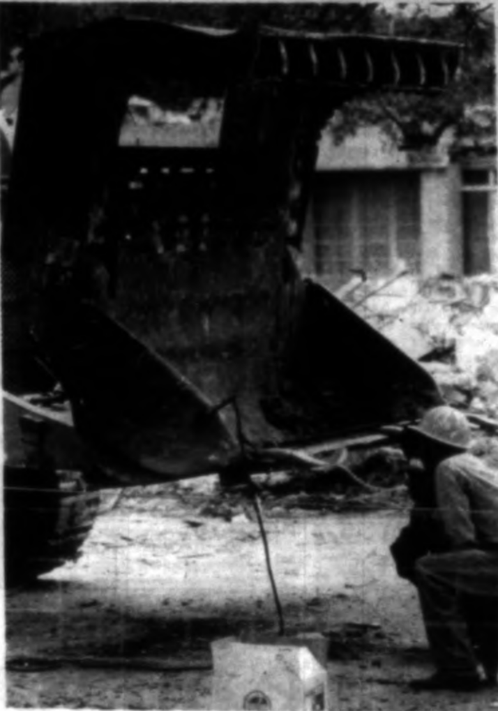
"OPEN WIDE, PLEASE?" fits this scene perfectly as workers examine a broken piece of equipment on a bulldozer cleaning up the rubble where the old MSC Post Office formerly stood. Cleanup of the demolished site is proceeding rapidly to make way for more renovation of the old MSC. (Photo by Gary Baldasari)
