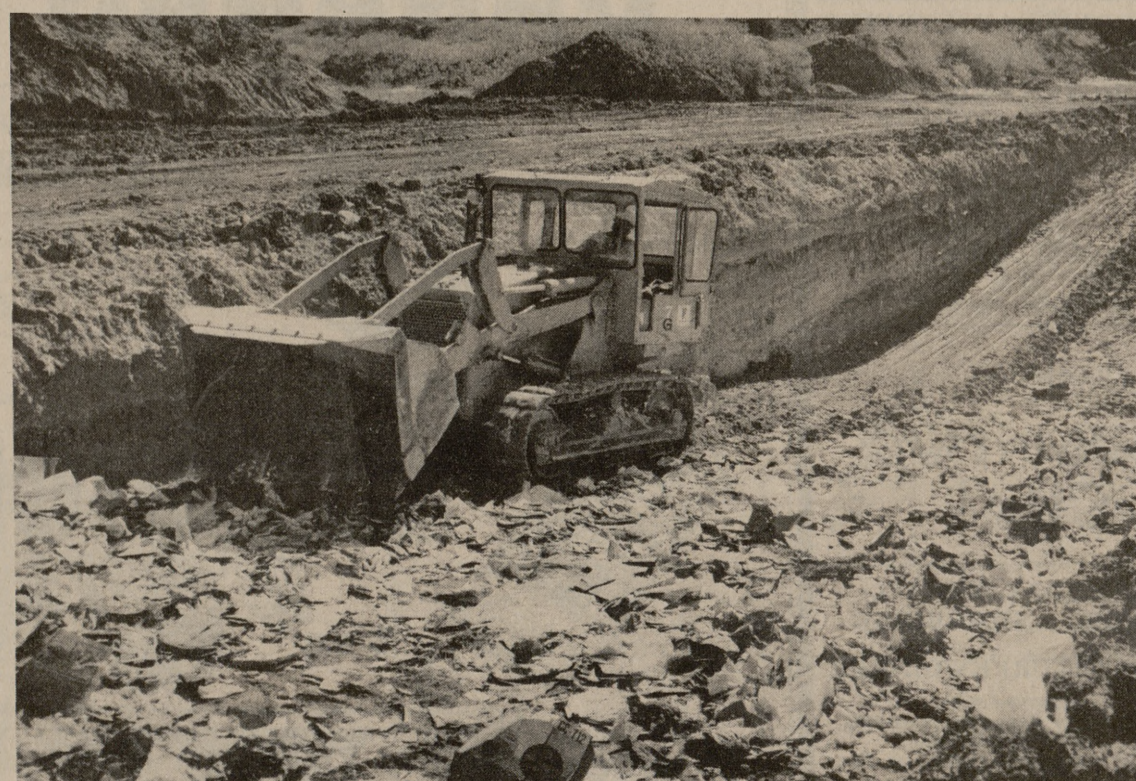
A CRAWL LOADER covers refuse at the 11-acre A&M sanitary landfill. The tractor has cut total operating costs in half, despite the 50 to 75 tons of refuse processed daily. About a foot of dirt is placed over the compacted trash.
