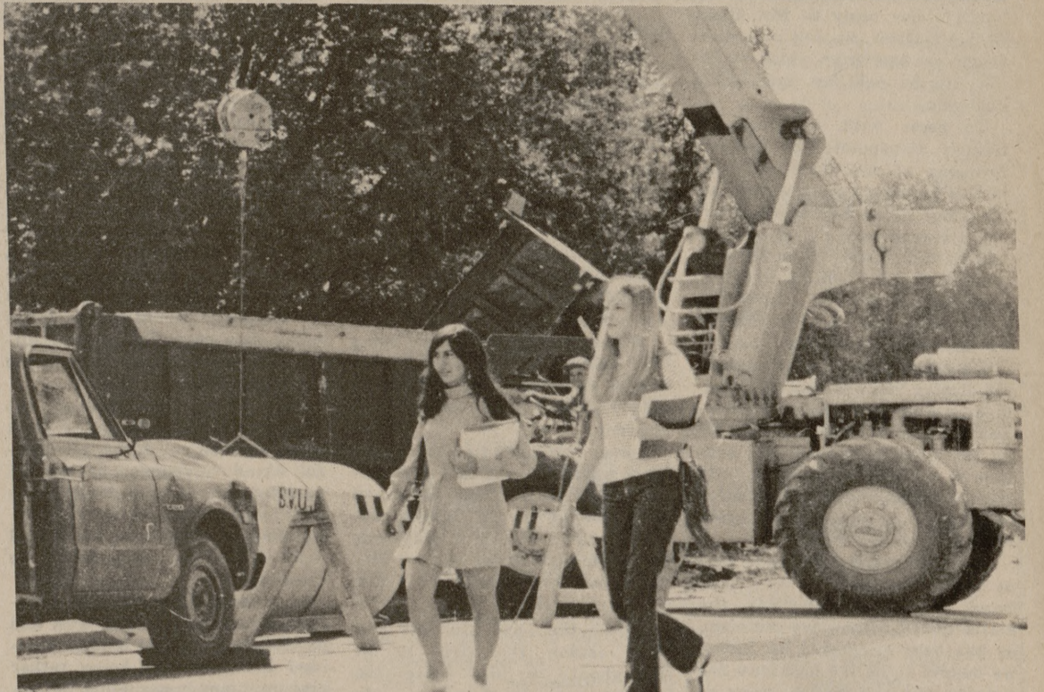
COEDS AND CONSTRUCTION are forced to put up with each other for the present as a storm sewer is being put in place in front of Dunn Hall. School officials claim most of the work will be finished by Oct. 14.
