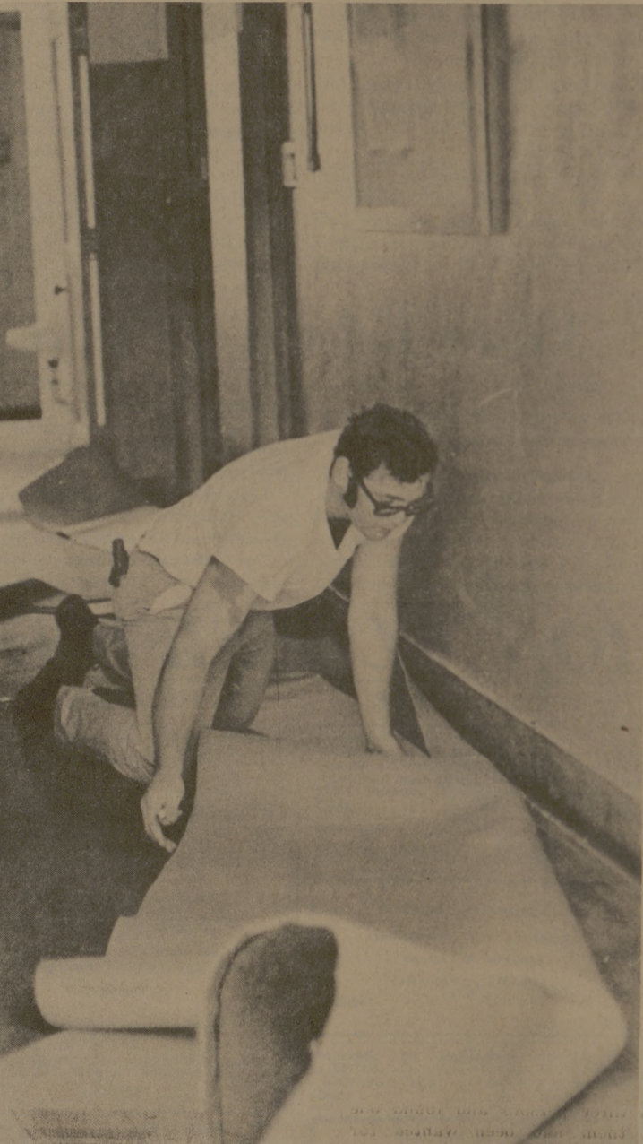
WALTON CARPET is being installed in all ramps in the A&M dorm as part of a dorm renovation program which received its blessing from last spring's Student Senate. Although some students are questioning the value of the carpet, Charles Hitzelberger is shown installing the carpet for the Walton residents. (Photo by Gary Baldasari)
