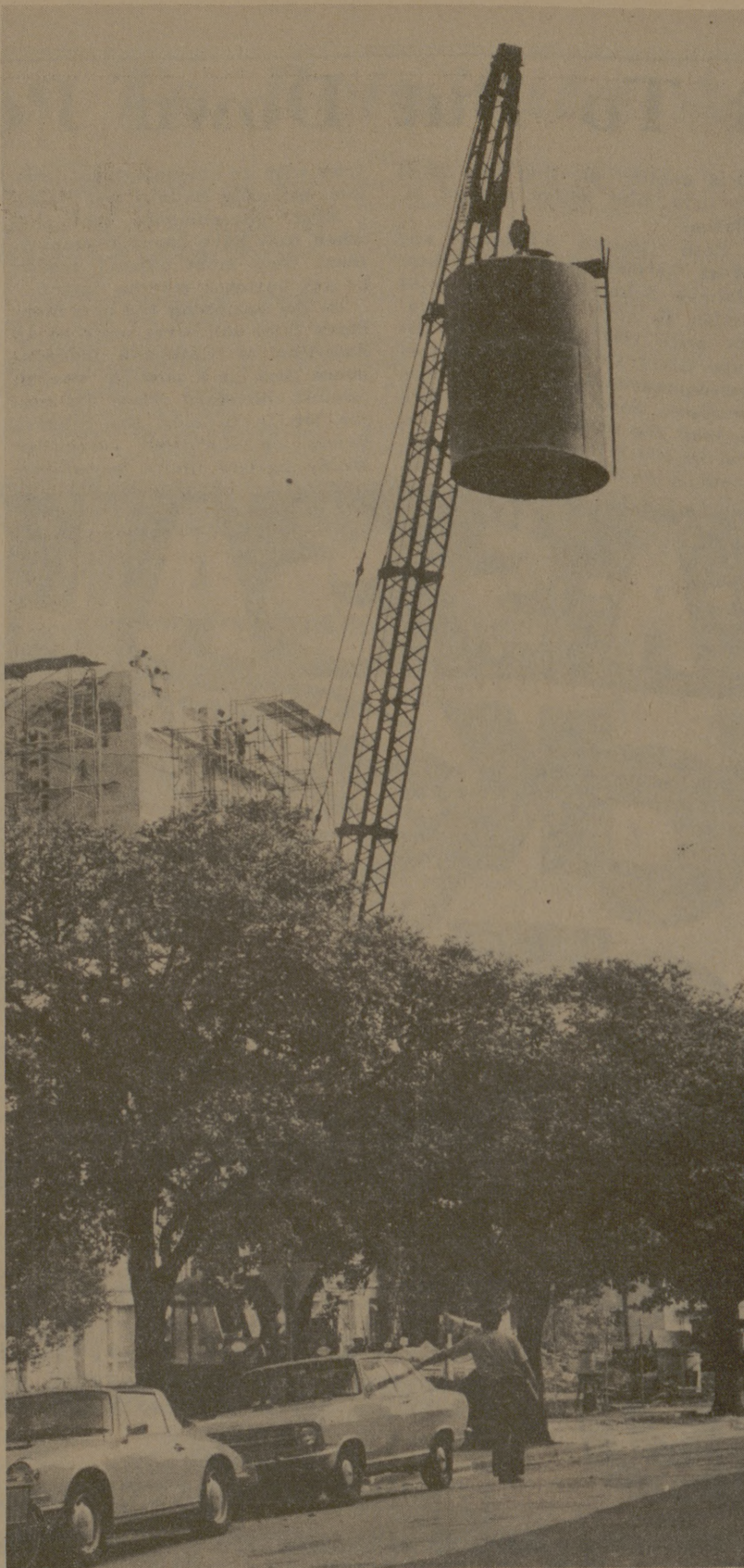
GEOLOGY TOWER DE-TANKED —A steel expansion tank around which the Geosciences Building tower was built in 1933 was removed Tuesday. Hot water used in the campus steam heating system was stored in the tank at one time. It was replaced by the power plant system about eight years ago.
