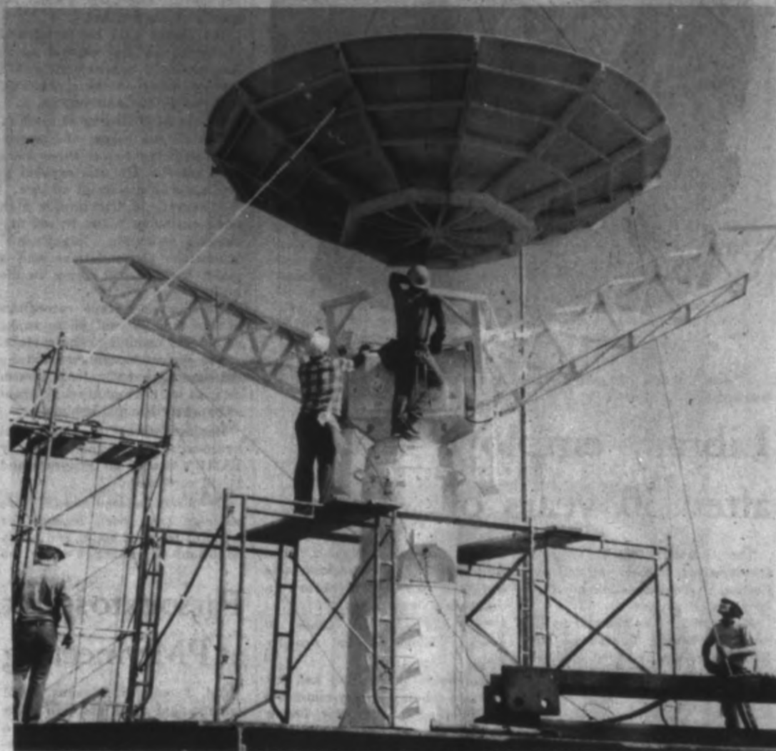
Workmen on top of the oceanography-meteorology building maneuver a 16-foot wide load onto the radar pedestal. Two five-foot-wide antenna were mounted on struts next to the main dish. A 240-foot crane with a 140-ton capacity was assembled by the Westheimer Co. of Houston for the installation.
