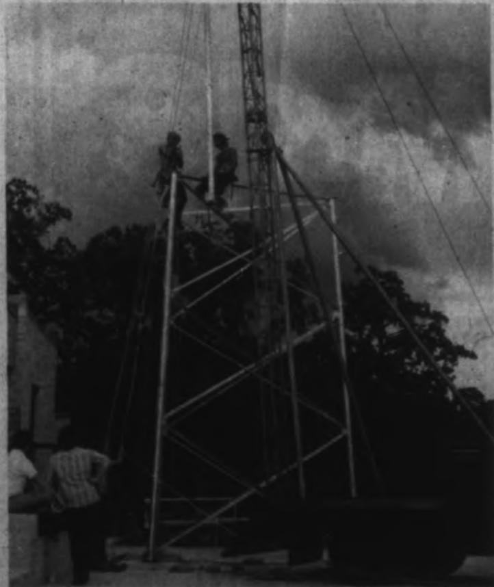
Microwave equipment carrying KAMU-TV signals from the Educational Television building to the station's transmitter-antenna site in Hensel Park will be mounted on this 100-foot tower.
