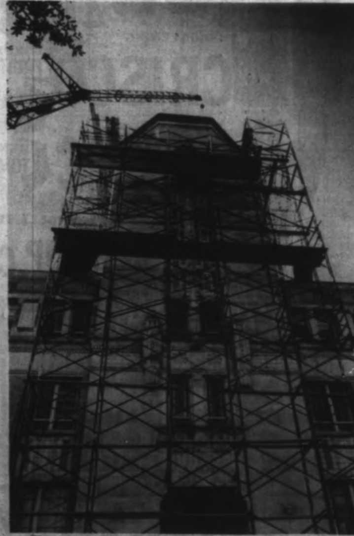
The tower of the Geosciences Building is being removed by workmen because it is a safety hazard. It has been a landmark since 1932. (Photo by Bob Leitz)
