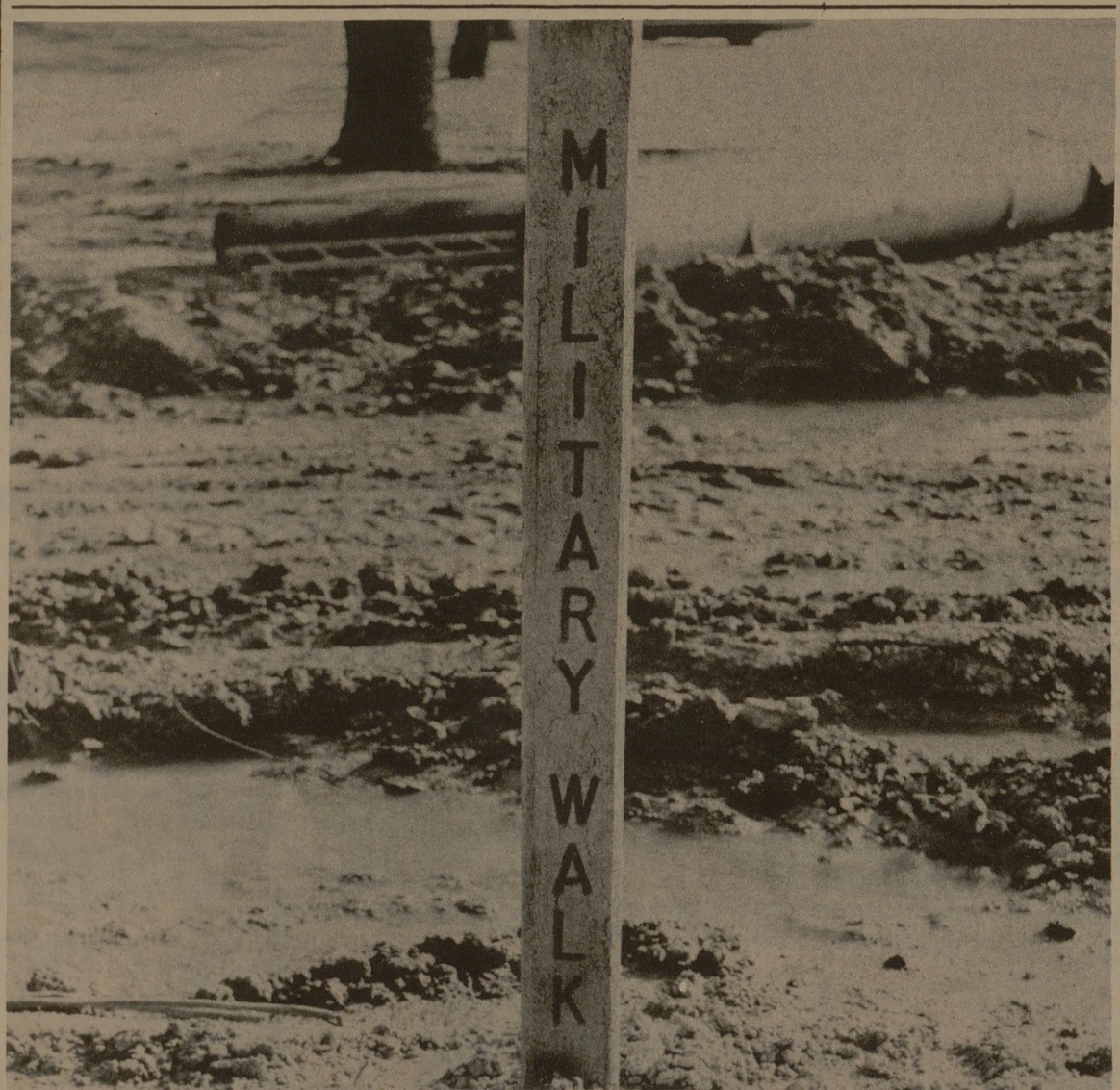
A SIGN OF THE TIMES at A&M is the Military Walk street sign in a bed of mud. The summer at Aggie land has featured a common sight, construction, and an unusual amount of rain, something not ordinarily in abundance from June through August. (Photo by Kenneth Stroebel)
