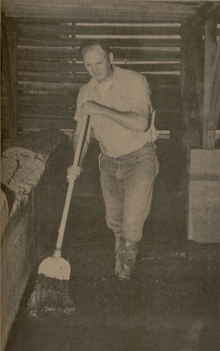
UGH! At least that is what this worker seems to be saying as he sweeps out the bottom of the cooling towers in the Physical Plant. The gunk is an accumulation of whatever falls into a cooling tower in 13 years—though we won't go into that. (Photo by Robert Williams)
