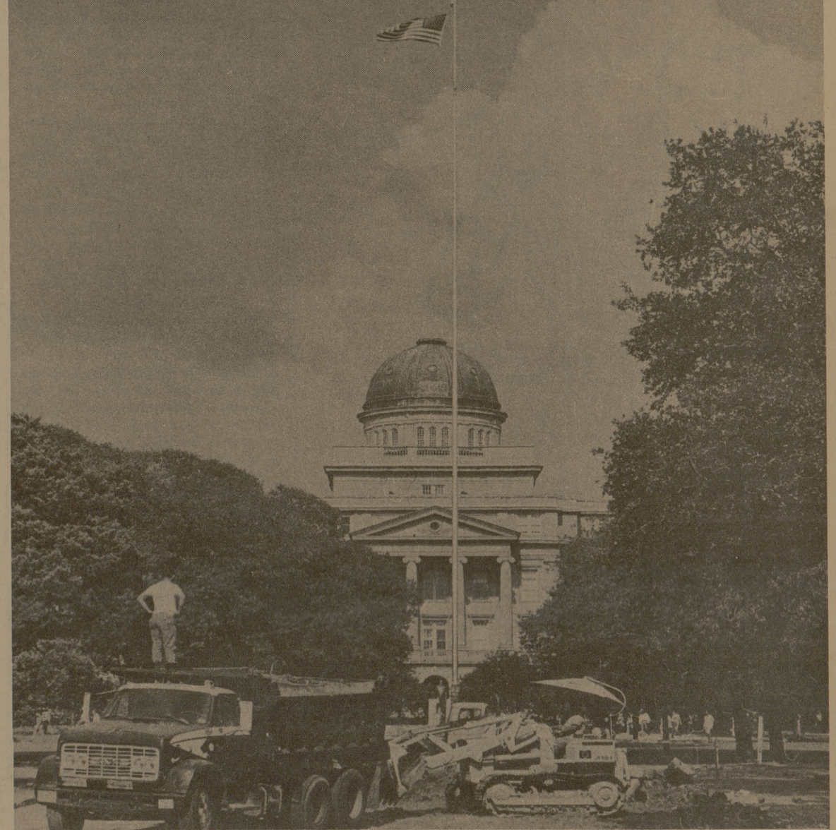
ANOTHER PARKING LOT takes shape between the YMCA and the Coke building, removing the north end of Main Drive. This action, plus the removal of several trees between the Coke building and the Meteorology building, has drawn criticism from students concerned about the environment and who gets to park in those spaces. (Photo by Hayden Whitsett)
