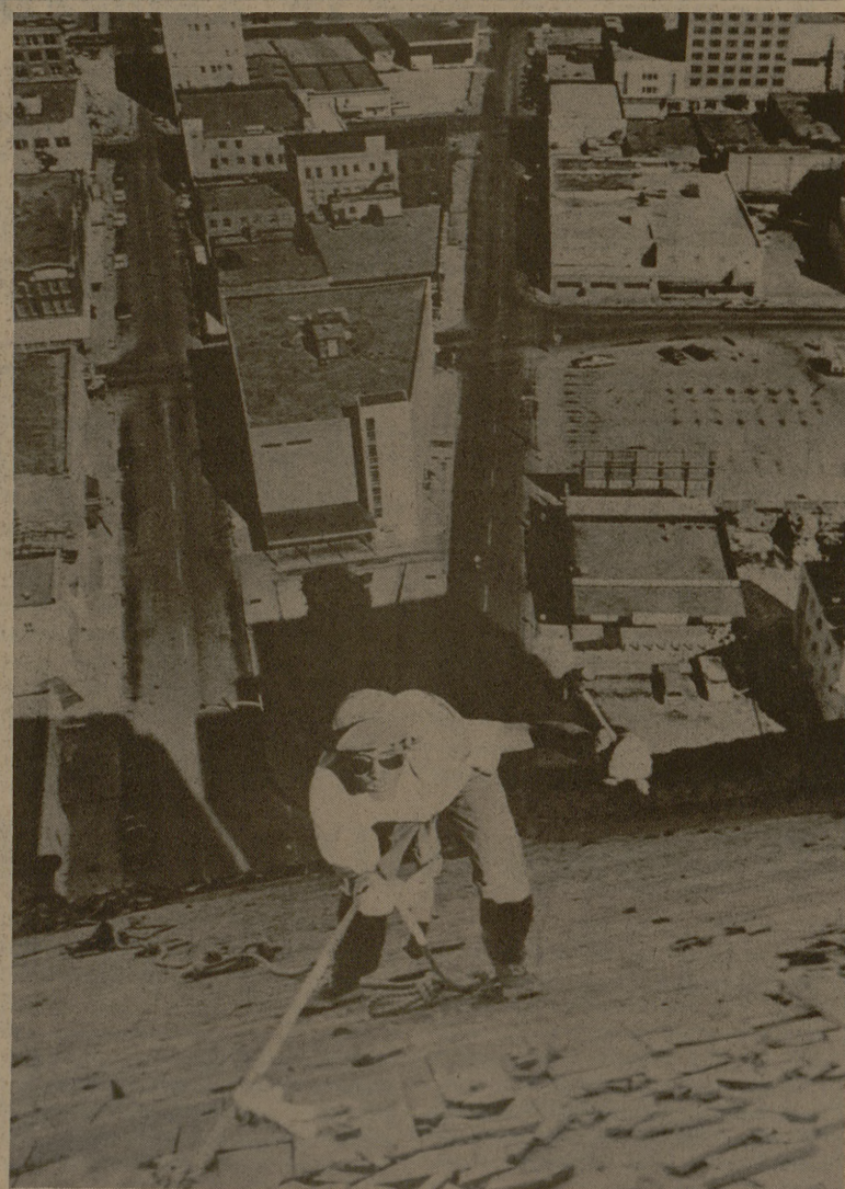
JOHN ROGERS LABORS atop the Driscoll Hotel several feet above earthbound passersby in Corpus Christi. Rogers is knocking roofing material off the roof of the now closed hotel which will be converted into an office building. (AP Wirephoto)
