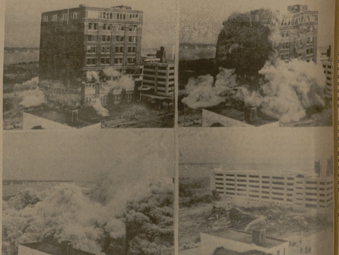
IN JUST SEVEN SECONDS, a series of dynamite blasts sent an eight-story building crashing to the ground in Memphis, Tenn. The demolition of the former cotton warehouse was by a Maryland firm that specializes in blasting away structures. No other buildings were damaged in the blast. (AP Wirephoto)
