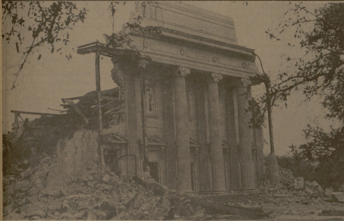
IT STILL STANDS. Olshan Wrecking Co. began razing campus landmark Guion Hall last Monday and predicted that the structure would be leveled last week. What remained Tuesday was piles of debris and the building's front, reminiscent of Green ruins. (Photo by Bob Cox)
