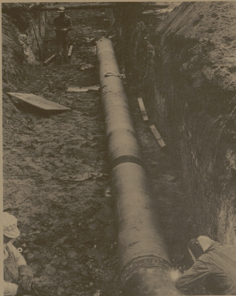
RAIN ALL DAY Tuesday didn't stop construction on the campus, even if it did get muddy in the multitude of holes. Welders continued on the pipe system being put in on the north side of the Academic Building, and the trench they were working in, about 10 feet deep, was no exception. (Photo by Hayden Whitsett)
