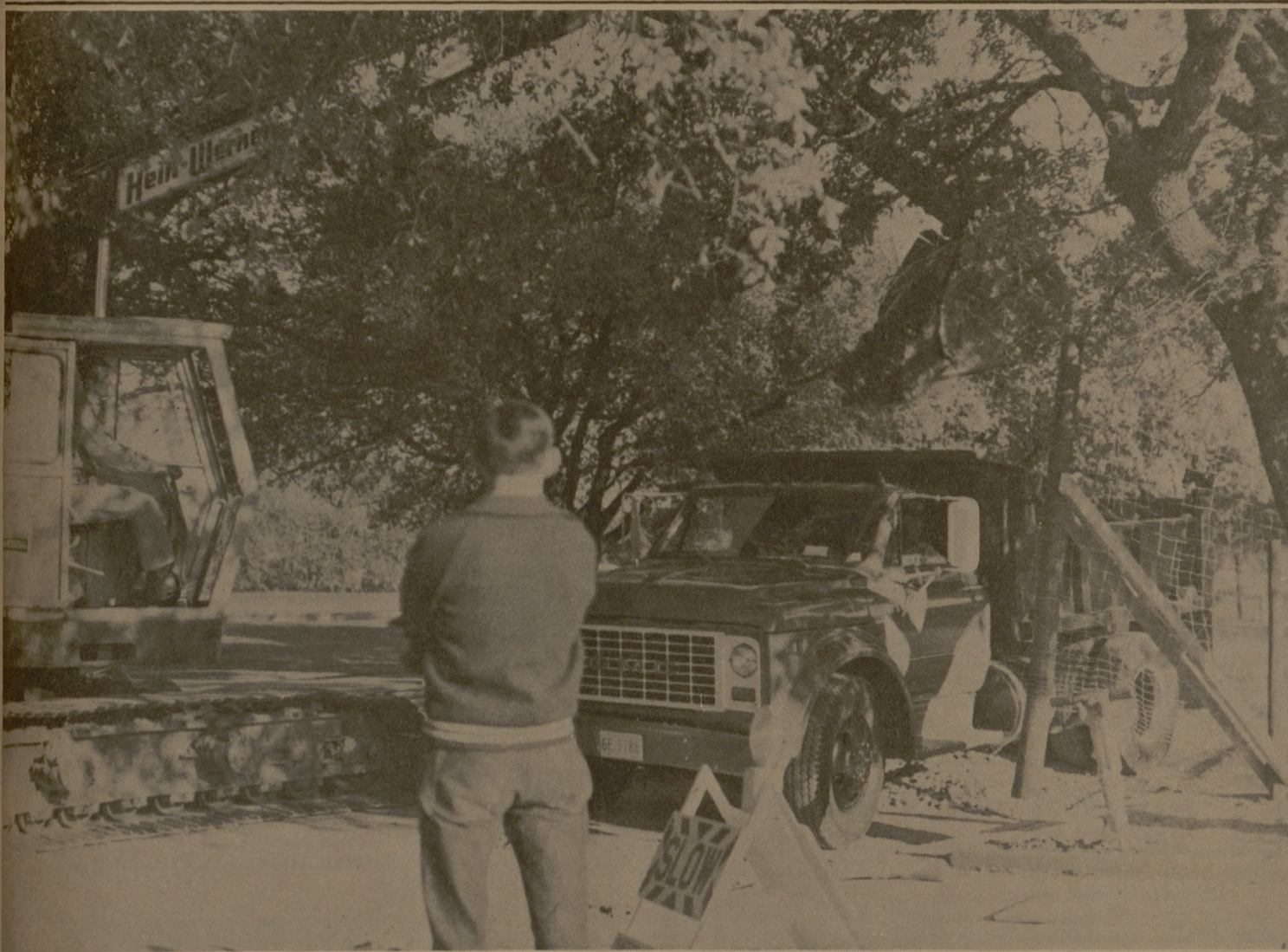
UTILITIES CONSTRUCTION between the Memorial Student Center and Guion Hall renders another section of the campus impassable to students and motor traffic. The work is both to install new utility pipes and begin work on expansion of the MSC. (Photo by Patrick Fontana)
