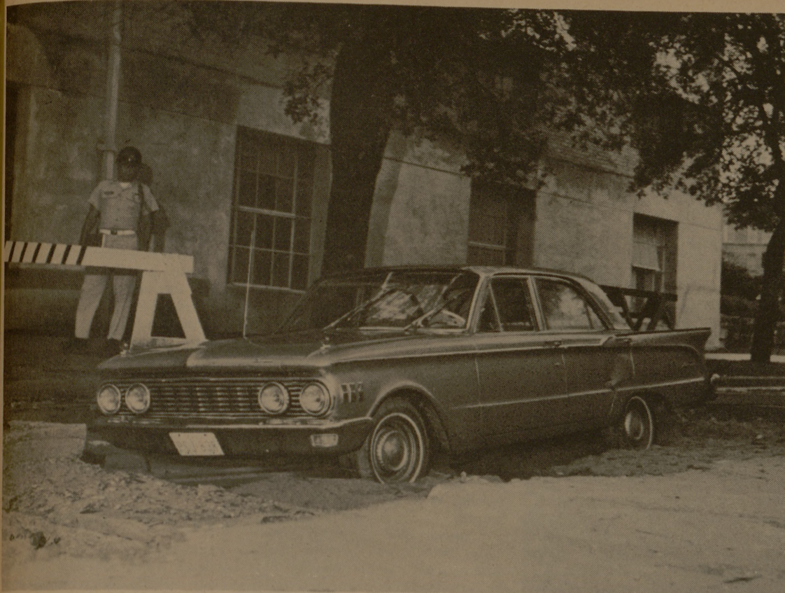
THERE WAS apparently some mix-up last night when a student drove down Ross Street into a recently filled ditch used in the chilled water line construction project. The right side of the car was dug out to chassis level in an attempt to remove it. Steve Lazaro, Houston junior, examines the problem.
