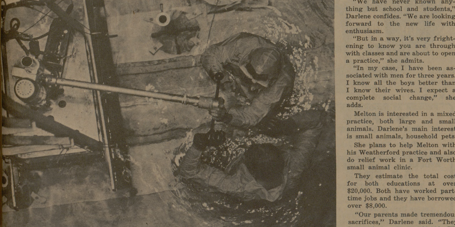
Inside nuclear reactor—Dr. John Randall and Dan Feltz of the Nuclear Science Center are shown inside the 40-foot nuclear reactor "swimming pool" drilling holes in the grid plate over the reactor core. The pool was drained to about five feet of water. A pre-drilled special overlay steel drilling plate was used to guide the electric magnetic-based drill in drilling the 12 one and three-quarter inch holes. Dr Randall is director of the center and Feltz is assistant director. (See story, page 4)
