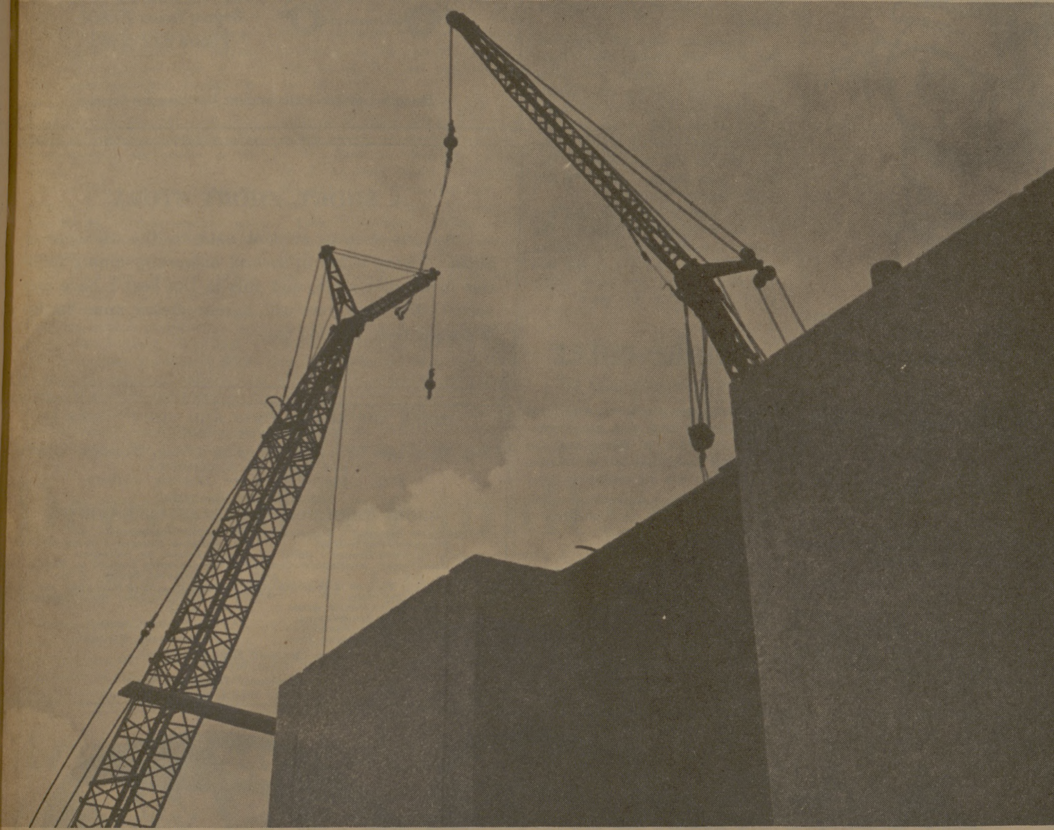
Huge cranes resemble giant insects over Engineering Center—$9.3 million building due to be ready for students next fall
