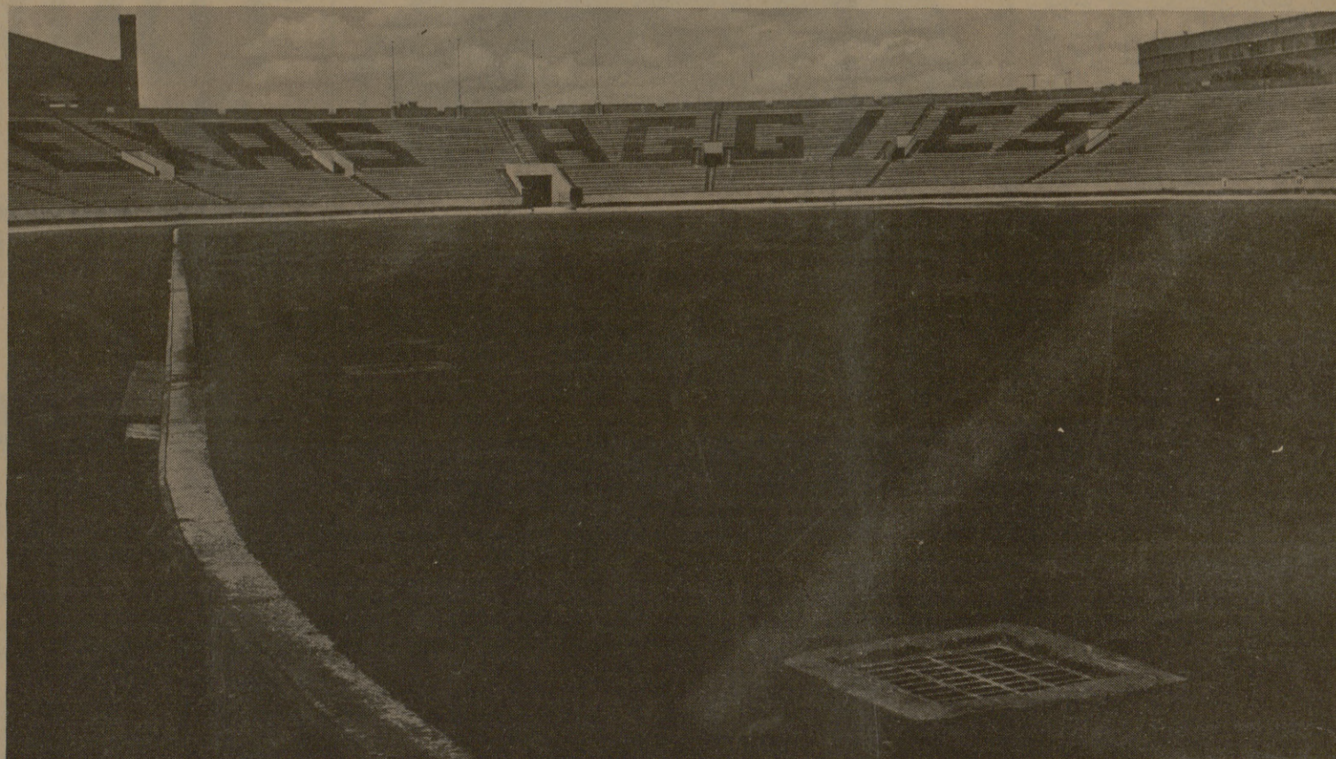
No parking lot this—Construction on Kyle Field's Astro-turf is coming right along as this photograph shows—the asphalt has been laid and next comes the glue. The arti-
