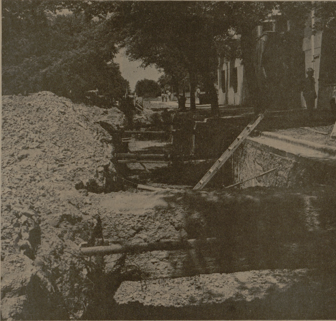
Construction underway—The construction being done on Ross Street is for a chill water supply and return line for a new dormitory. Other construction is for the extension of the sewer system. (Photo by Pat Little)
