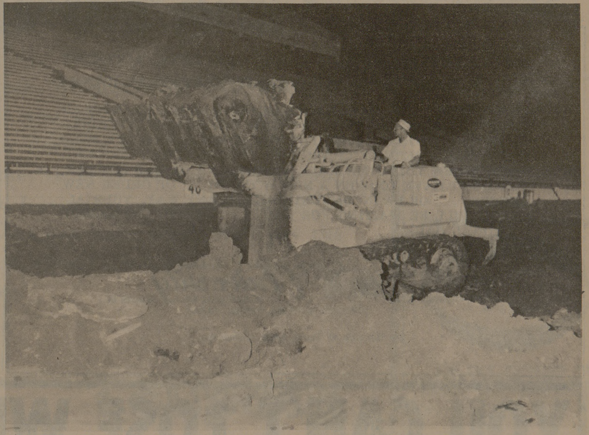
NIGHT DIGGER—Workmen continue to dig out portions of Kyle Field turf Thursday night, trying to remain on schedule for the installation of AstroTurf on the playing field. A Tartan track will also be installed in the stadium. (Photo by Mike Wright)
