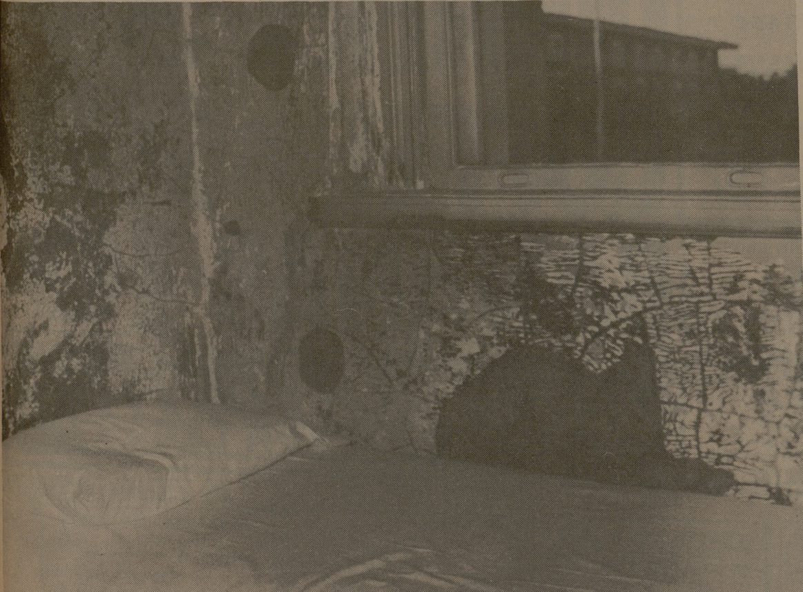
DEPRESSING SCENE The walls of a room on the second floor of the University Hospital show the ill effects of weather. Moisture seeping through the walls or leaking from the roof, hospital authorities say, causes the paint to crack and peel. They also say that repainting is a futile attempt. (Photo by Pat Little)
