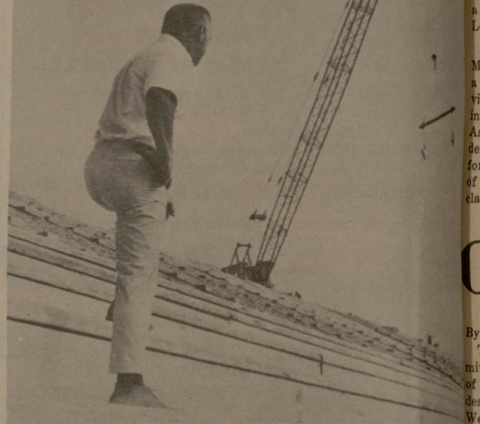
TEXAS INTERNATIONAL Leo Margolian, general manager of the Texas International Speedway, watches completion of the grandstands for the first Can-Am race scheduled for Nov. 9 at the $8 million structure.
