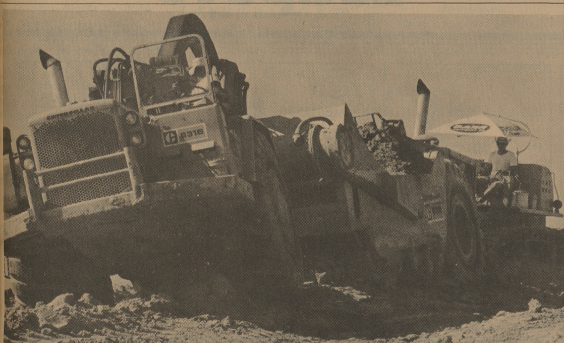
CLEARING THE WAY Work on the new Texas International Speedway moves along as workers from the Holloway Construction Company clear land for the project. The construction company has the cut and fill contract for the speedway, and has cleared about 300 acres so far. (Photo by Bob Stump)
