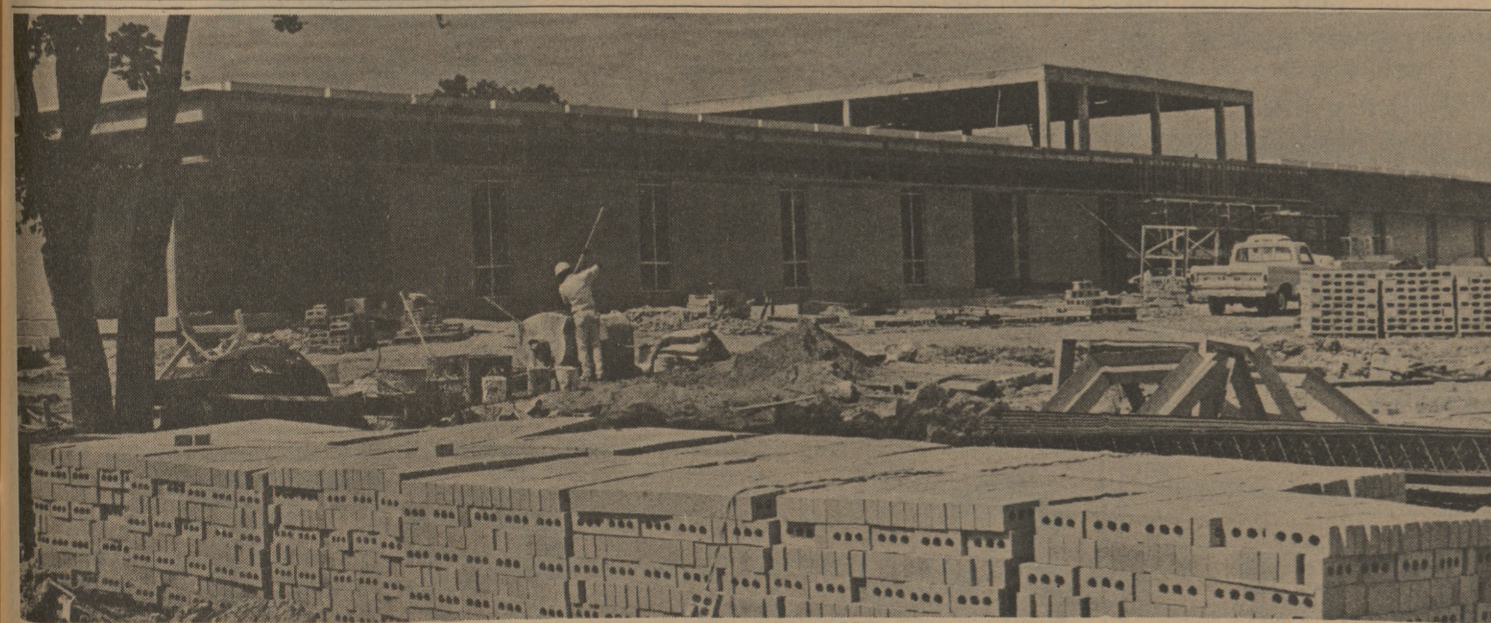
ONLY ONE OF NINE Construction continues on the A&M Animal Toxicology Research Center, one of a nine-building complex being built west of College Station. (Photo by Bob Stump)
