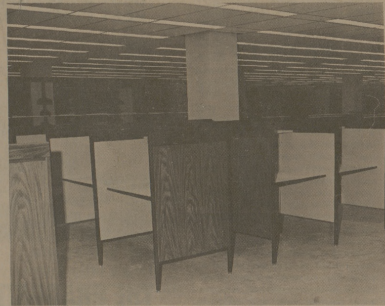
Once the parts are inside, they are installed in place. Electronic learning aids, recently demonstrated at the Educational Television Department here, are to be added later. (Photo by Mike Wright)
