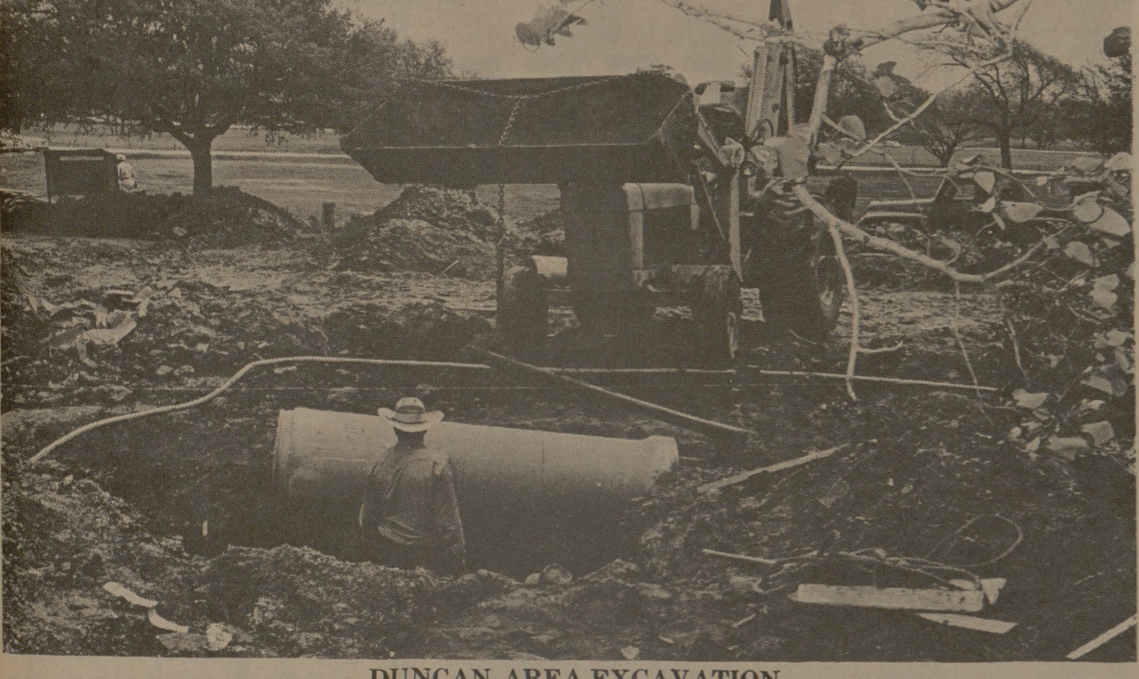
DUNCAN AREA EXCAVATION Workmen supervise the lowering of a drain pipe between Dormitories 5 and 7 in the Duncan area. The scene has been repeated recently throughout the area as work begins on inter-dorm lounges. (Photo by Mike Wright)
