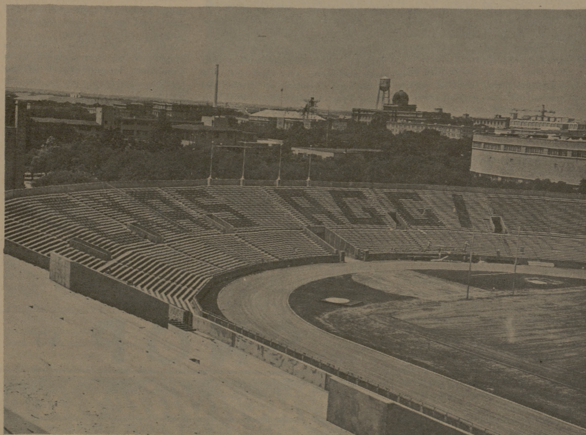
T-E-X-A-S A-G-G-I . . . The north end zone of Kyle Field is given a new look as construction work on the stadium continues. The new white and maroon bleachers being installed will spell out "Texas Aggies" when completed.
