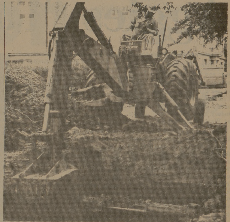
ARM OF CONSTRUCTION Work continues along Military Walk behind the YMCA. Laying of the air-conditioning pipes will necessitate a temporary blackout over the weekend in several buildings along the "Walk," including Sbsia Dining Hall.
