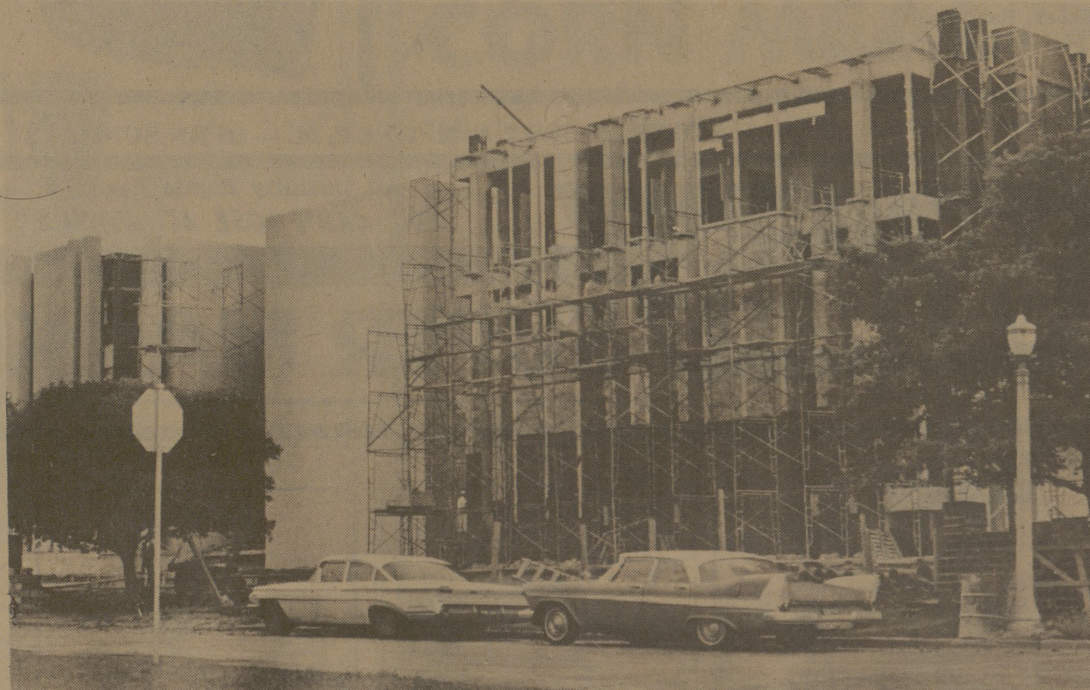
CONSTRUCTION FOCUSES ON THE FUTURE . . . NASA's $2.25 million Space Science Center near completion.
