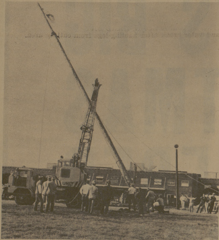
CENTER POLE GOES UP ... Spider D members put center pole in place.
