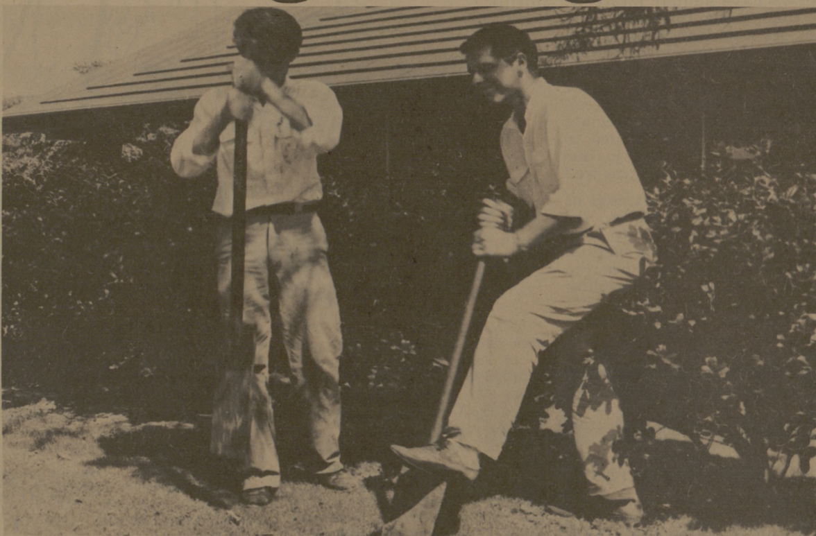
A HARD DAY'S WORK Lewis Elliot, left, and Billy Burt of John Watson Co., lift turf to lay electrical conduit that will carry power lines for the con-
