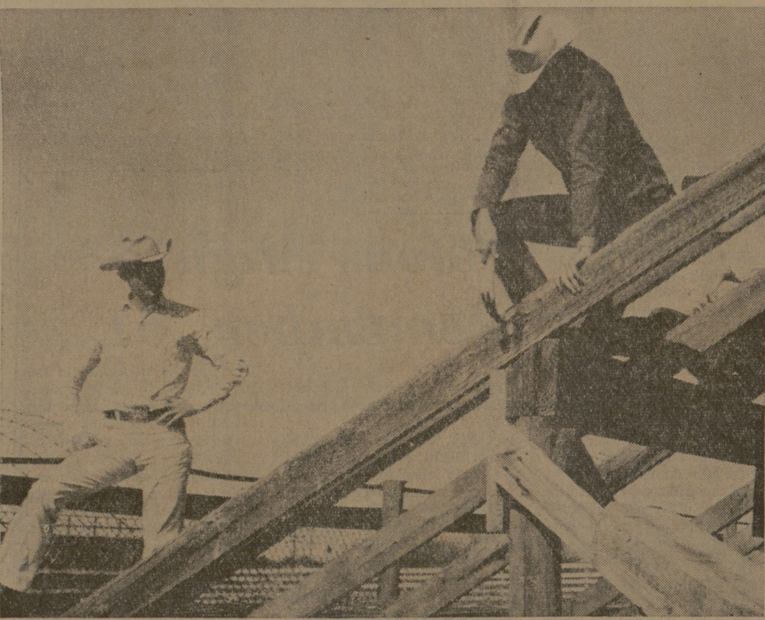
Rodeo Arena Undergoes Repairs Pounding away with hammers during rebuilding work on the rodeo arena are two members of the Rodeo Club and Saddle & Sirloin Club, Britt Jarvis (right) and Bobby
