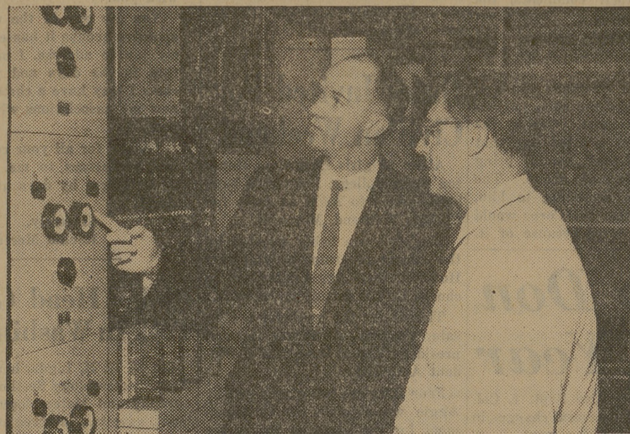
Roy Vaughn (left) discusses a central office power installation with Switchman R. F. Heider.
