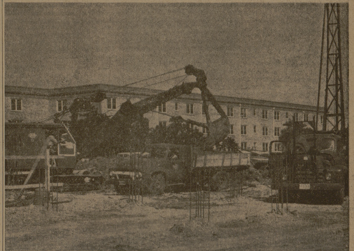
JUNCTION MANOR TAKES SHAPE as the construction crew clears the ground and sinks the foundation piers. On this spot Aggie footballers will soon have a "home of their own."
