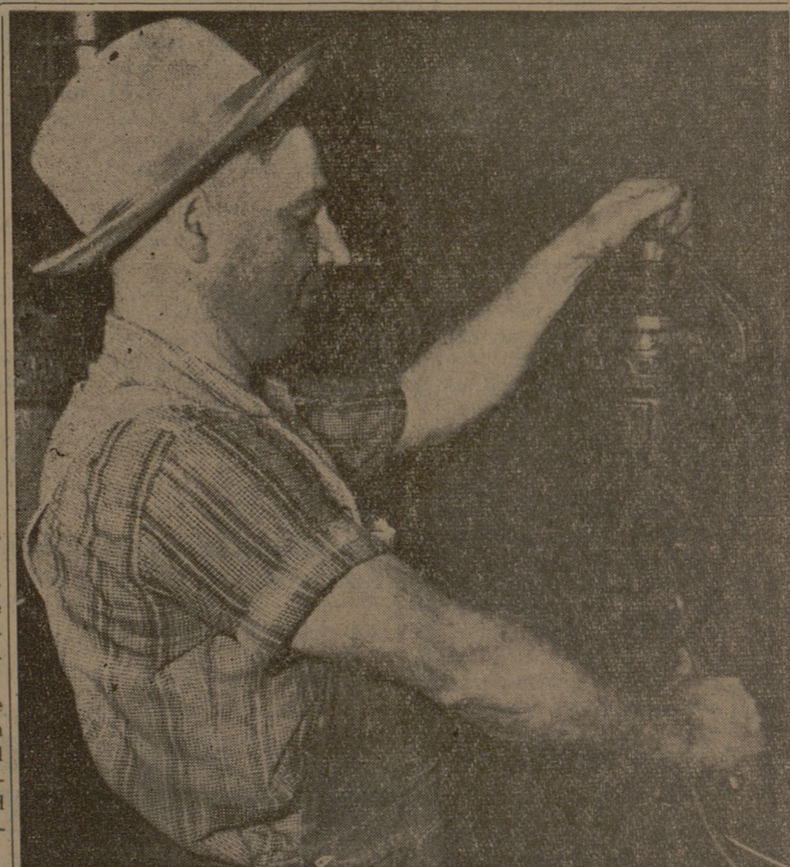
TIGHTENING THE LAST BOLT on one of the fuses in the electrical junction box in front of Duncan Mess Hall which was short circuited Wednesday night is George Carroll, of the B&CU Department.
