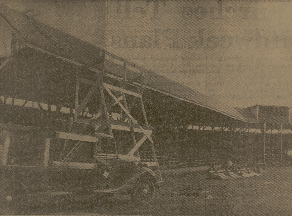
NEW ROOFING ON KYLE FIELD —Repair work in the shape of a new roof on the Kyle Field baseball stands nears completion. All repairs were made by A&M and the new roof offers better protection and a neater appearance to the park which had recently become shabby.
