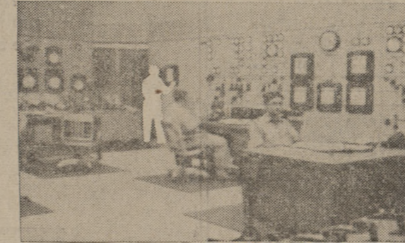
System Control for Utilities
