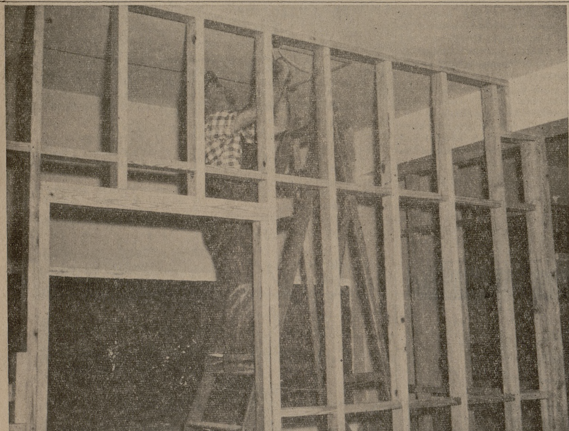
REMODELING NAGLE HALL—Assuming a new form under the hands of the carpenters to become the home of several departments of the School of Arts and Sciences. Here is a section of the basement which will house new quarters of the Journalism Dept.
