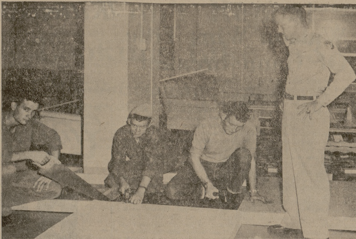
MORE LOUNGE RECONDITIONING—Roy Lackey, Sam F. Ray, Bob Hoover and John F. Heard are shown above (left to right) working on the new additions to the lounge in Dorm 9. All walls are being repainted, ceilings lowered, screens placed about the door and phone; this work is scheduled to be finished Nov. 1.
