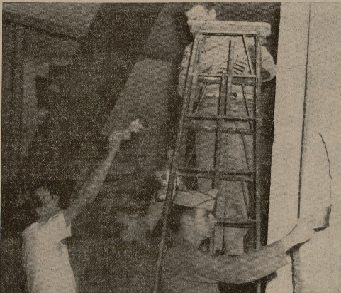
HARD AT IT —Shown above (left to right) Joseph Donaldson Jr., architecture instructor; Wade Driver; Norman Ufer and Mike Talley are painting the inside of the dome of the Academic Building. It is to be made into an architecture classroom.
