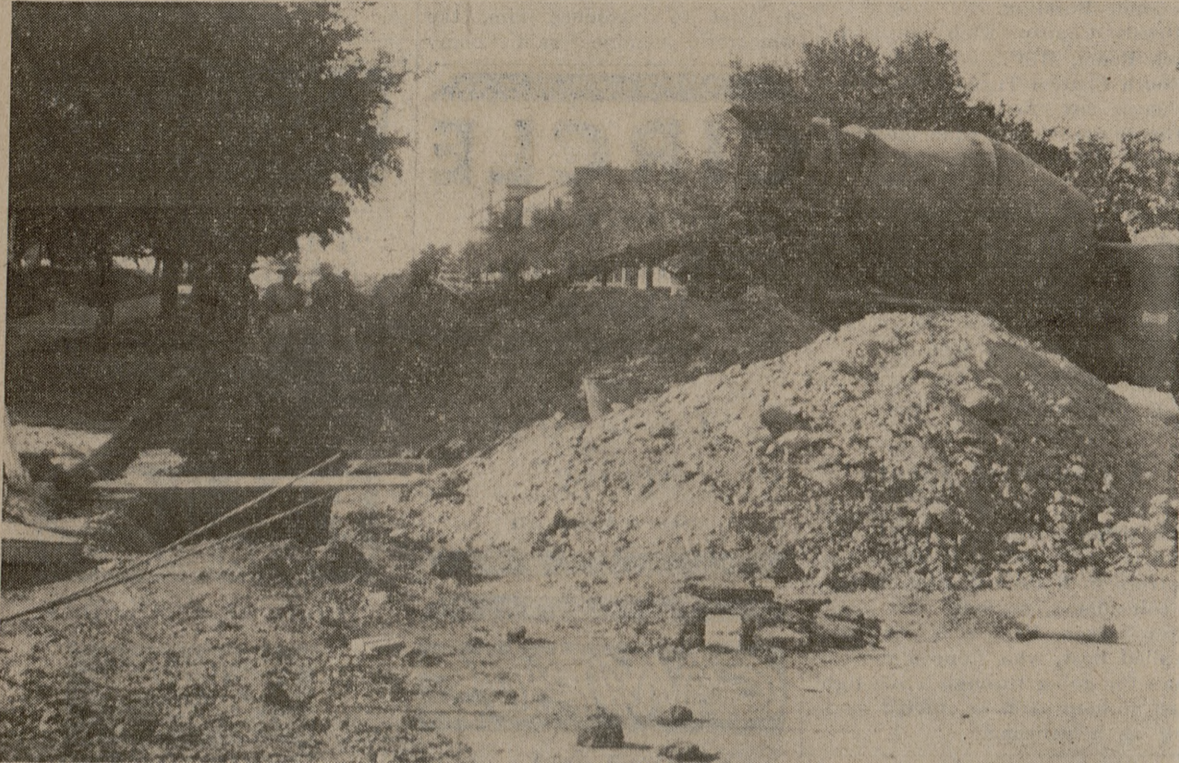
IT HAPPENS EVERY FALL—Workmen are pictured putting down an electrical conduit system on Nagle Street. The system will serve the new Dairy and Biochemistry Building.
