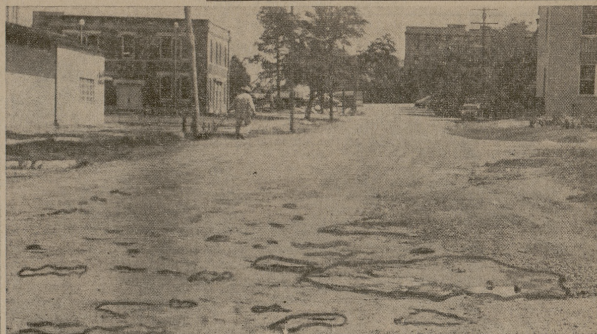
ONE OF A&M'S "HOLY" STREETS —Scheduled for early repair, this scene is typical of the condition found when traveling down Nagle St. which runs beside the A&M Press Building down by the Shack Area. Now in axle-breaking condition the street is shown being traveled by a wise man—on foot.
