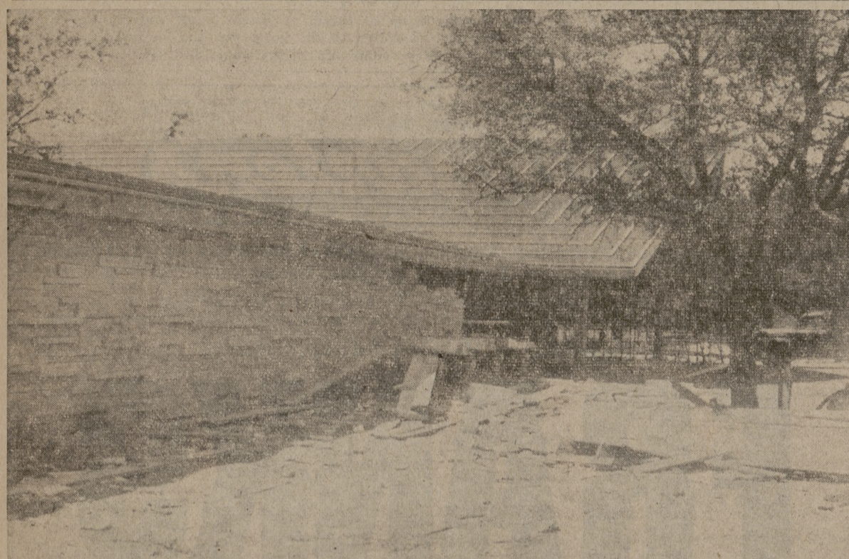
THE CHAPEL —A&M's new chapel, made possible by the Former Students Association nears the halfway mark in construction. Richard Vrooman of the Architecture department designed the building.
