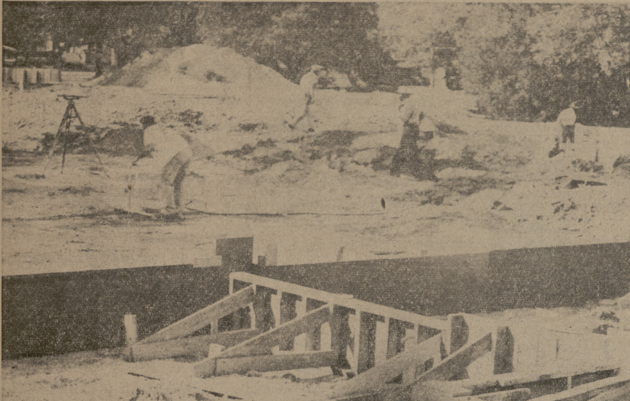
CHAPEL CONSTRUCTION UNDERWAY —The new A&M Chapel, made possible by the Former Students Association, progresses as scheduled. Workmen this week completed setting first stages of foundation for the new structure.
