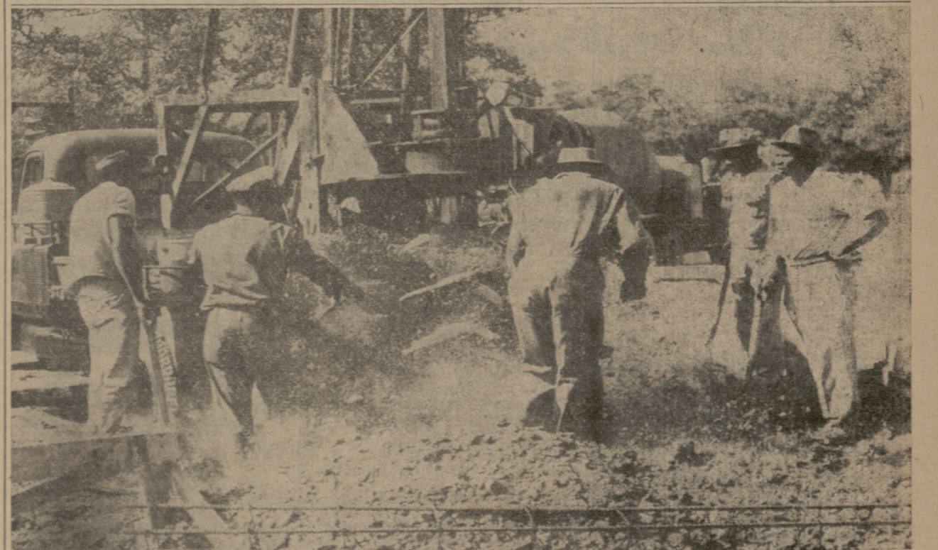
GOING DOWN—Workmen stay away from flying dirt as work progresses on the foundation for the new A&M Chapel. The building is being constructed by the R. B. Butler Construction Company of Bryan, and will be located on the northeast corner of Houston and Jones Streets, across from the President's home and immediately behind Law and Puryear Halls.
